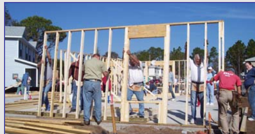
Apostle's work together to raise a wall on the first day of construction.
